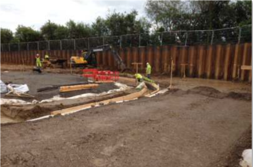
Construction of new access road for the car park and service yard in progress
