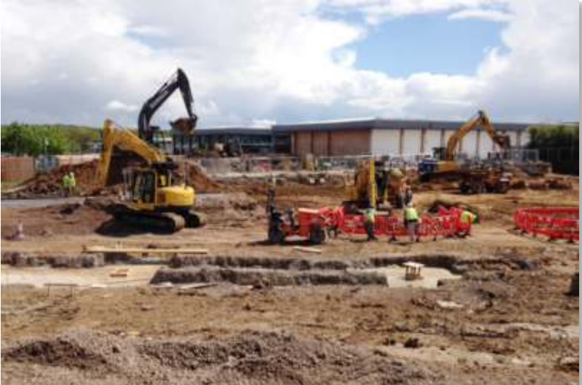
During May the main bulk excavation has been completed, and foundations for the new cinema commenced
